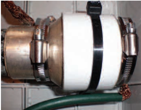
PHOTO 7: Detail of the connections to the capacitor.
